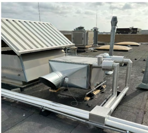
One of two Lepidos installed at CWS Workwear
