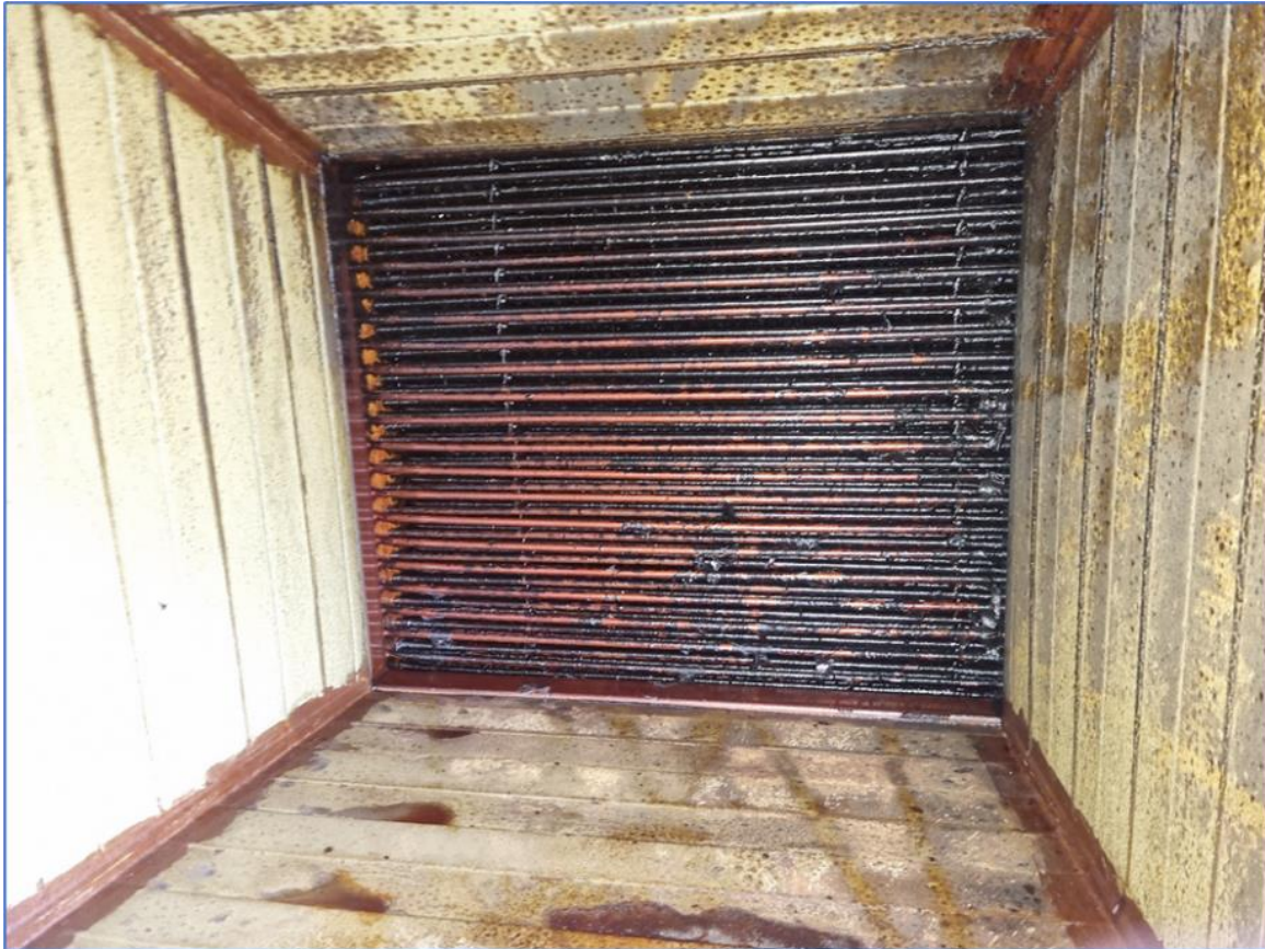
Figure 4. Photo of the inlet side of the exhaust air into the Lepido after 22 months of operation without pre-filtration or ongoing maintenance
